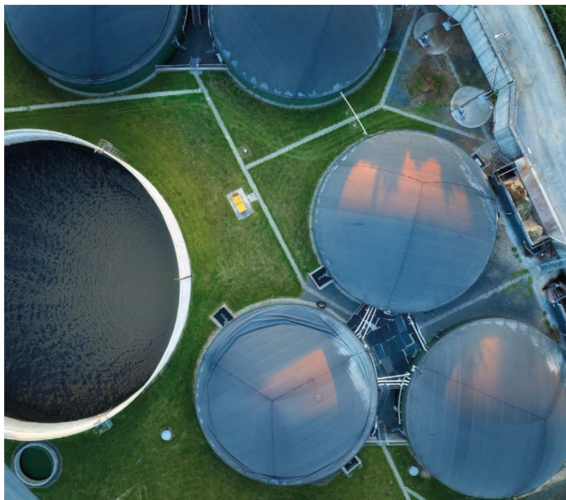
Process components, fermenters and biogas storage tanks
